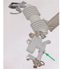
S&C Fault Tamer Fuse - Open
